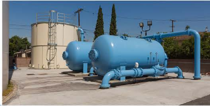
Maywood Mutual Water Company No. 1 Maywood, CA 1,000 GPM Iron and Manganese Removal System
