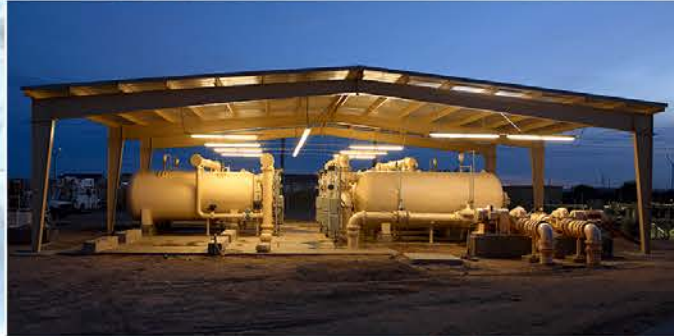
Sundance Water Treatment Plant Buckeye, Arizona 5,000 GPM Arsenic, Iron and Manganese Removal System
