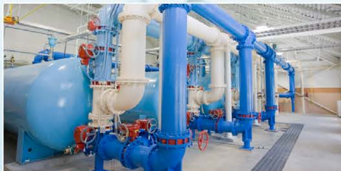
City of Fredericton New Brunswick, Canada 4,755 GPM Iron and Manganese Removal System
