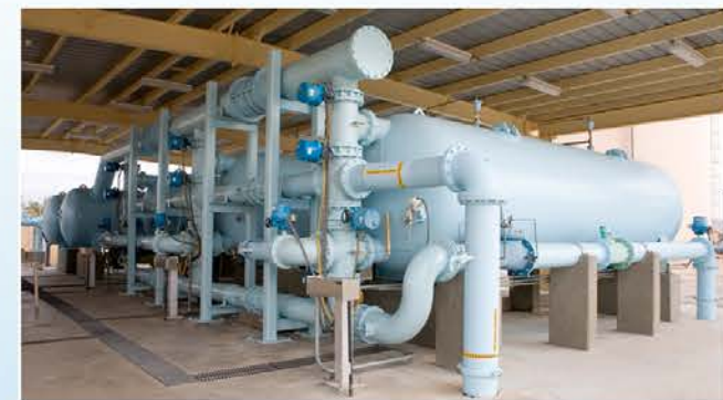
City of Yuma, Arizona 6,000 GPM Iron and Manganese Removal System AWPCA 2005 Water Project Of The Year
